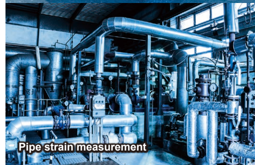
Brake and pipe strain measurement
